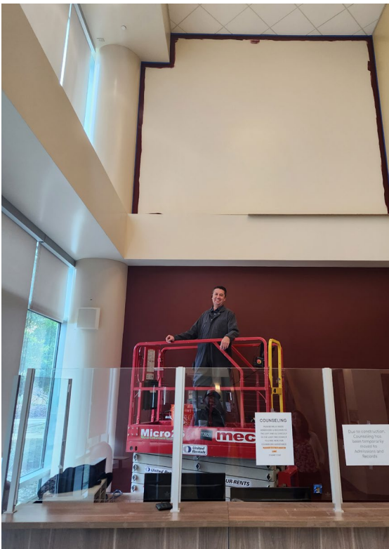
What a rock star! Jon Garner, Director of Facilities was captured adding color to the wall that will eventually become the new Welcome Center inside the Records and Admissions building. Thanks Jon!
